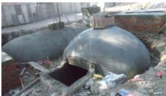
Rysunek 5 Bioreaktor w trakcie budowy. Źródło: Health care waste management towards the circular economy: a case study at Tribhuvan University Teaching Hospital in Nepal
